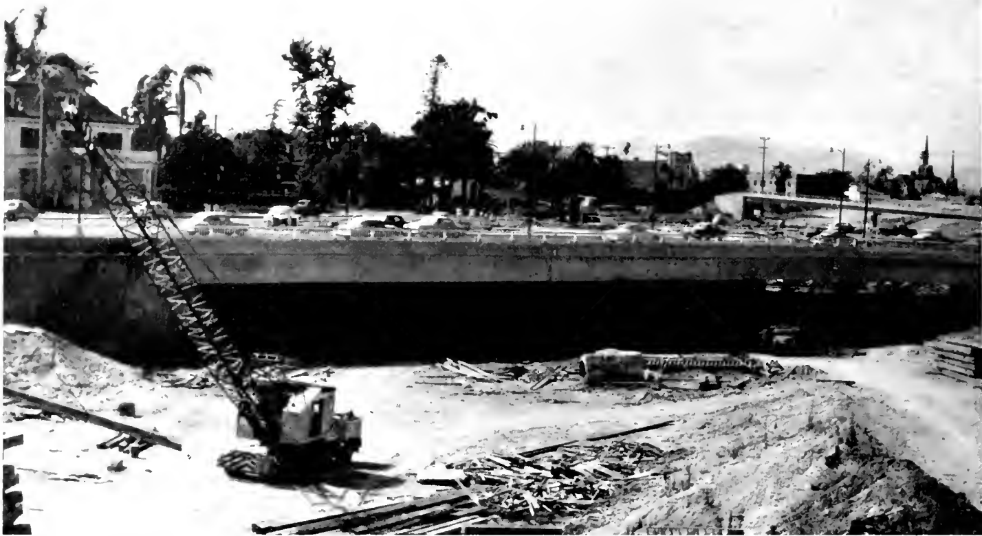
Looking northwesterly along Harbor Freeway construction, showing nearly completed Figueroa Street bridge at 23d Street
